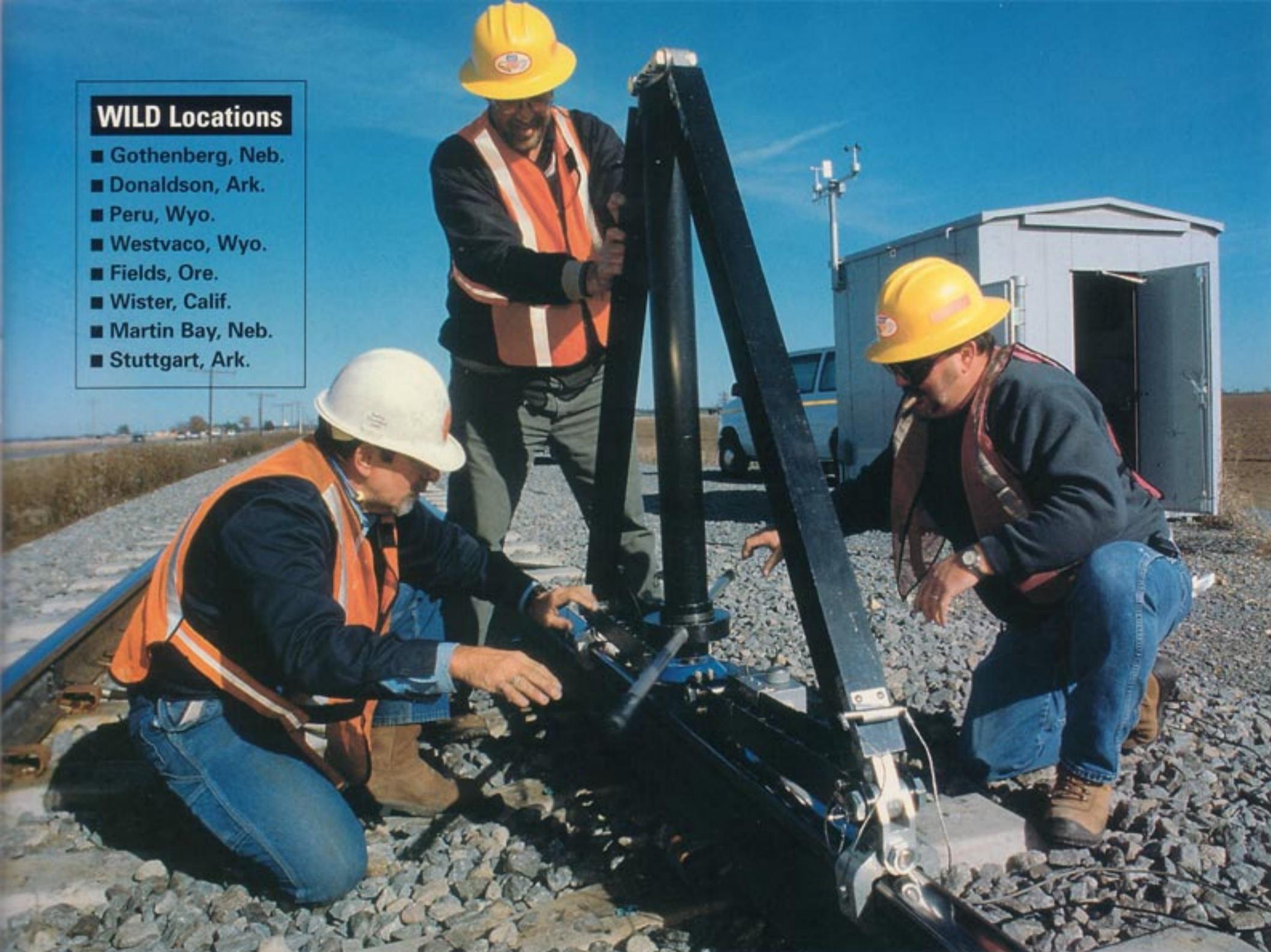
Using an A-frame fixture to calibrate each of the WILD's 32 measurement zones in Stuttgart, from left, are Signal Maintainer Chuck Shock, Engineering Manager Bill GeMeiner and Hastings.
